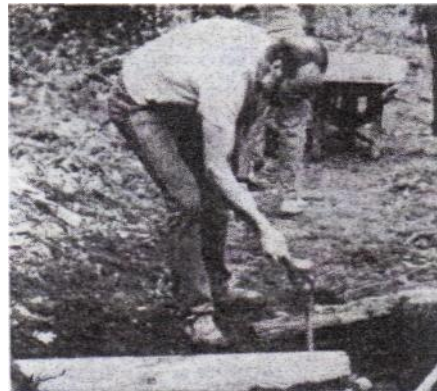
Jeff Windeshausen installs a water bar during a trail maintenance work party. Volunteers report getting personal satisfaction from such volunteer work.
